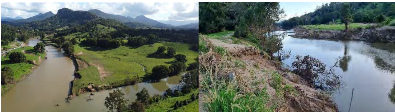
Photo 7-4: Drone photo – bank erosion at the confluence of Tweed and Oxley Rivers (left); bank erosion on the Tweed River following the March 2002 flood (right). Source: Submission to the Inquiry from Neil Baker.
