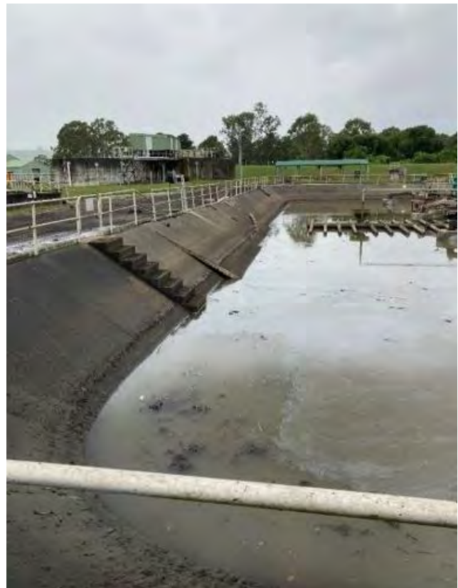
Photo 3-9: East Lismore STP damage. Source: Public Works Authority.
