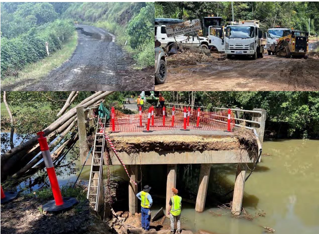
Photos 7-3: Flood-damaged roads and bridges in the Northern Rivers Region. Sources: Mrs Debra Van Den Berg, submission to the Inquiry and Mr Daniel Strzina, submission to the Inquiry.
